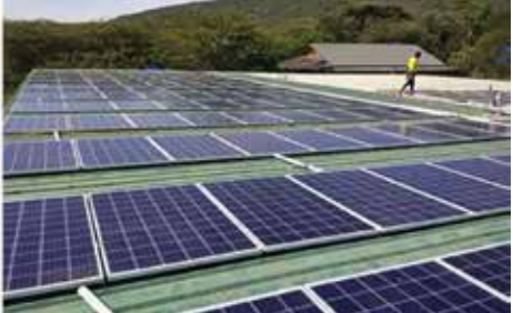
Nanyuki Commercial PV System CAPACITY: 100Kw Nanyuki
