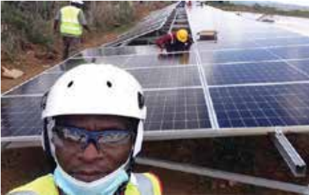
Roof Mount System CAPACITY: 600 KW Naivasha
