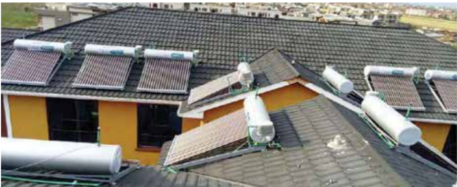
Solar Water Heating System CAPACITY: 6400 Liters Dorothy Park Langata By Sekandi Holdings
