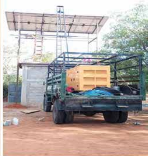
Solar Borehole Water Pumping CAPACITY: 4Kw Emali, Makueni
