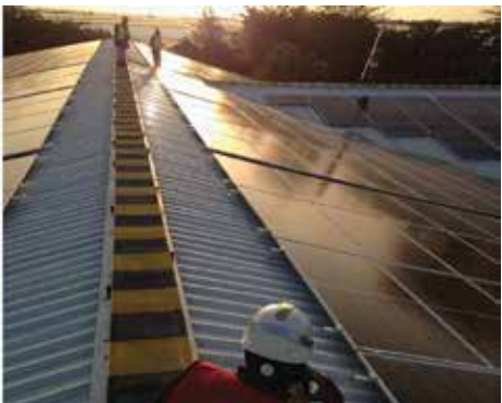
100Kw Roof Mount System Nairobi
