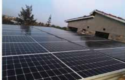
Kamulu Solar Water Pumping System CAPACITY: 15Kw Kamulu
