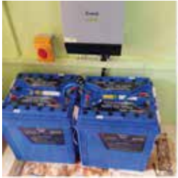
Residential Power Backup CAPACITY: 5Kw Karen Hardy
