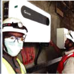
Residential Hybrid 3 Phase System CAPACITY: 10KW Nairobi
