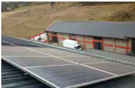
Common Area Solar PV CAPACITY: 5Kw Kenol Muranga
