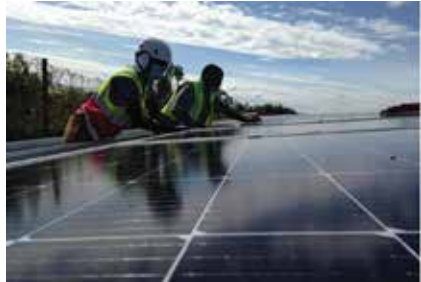
Roof Mount System CAPACITY: 600 KW Naivasha
